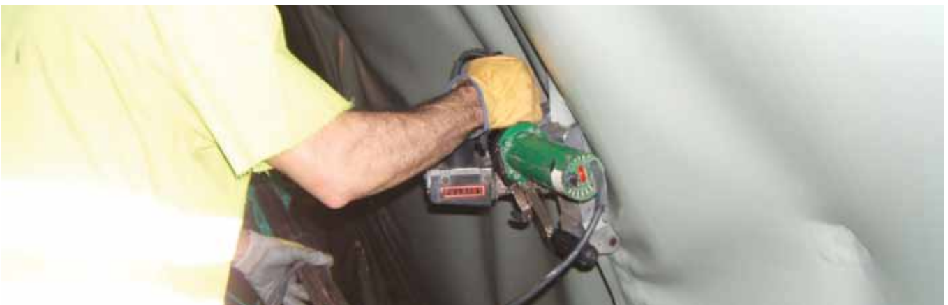
The geomembranes are welded together with automatic welding machines producing a seam with testing canal.
