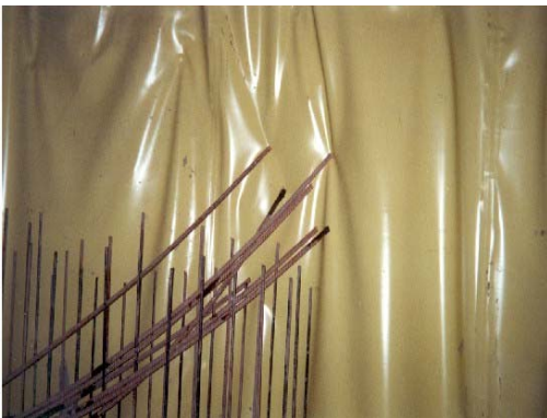
Reinforcement bars endanger geomembrane
